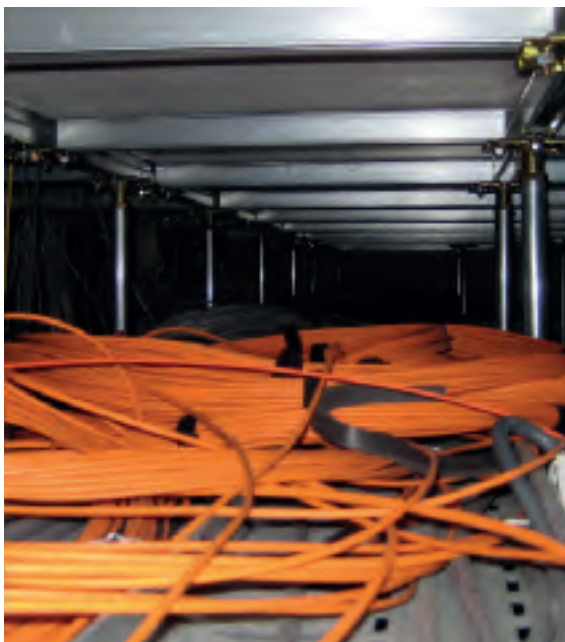
Figure 3. Cramped, inefficient data IT shed.
